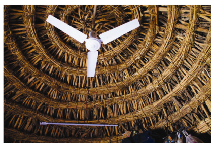
Fan and tube light inside the home deployed with inverterless system.
