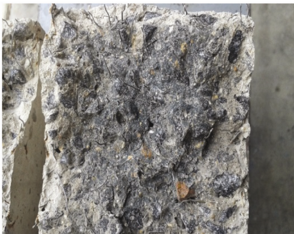
Figure 6. Typical failure surface of the beam.
