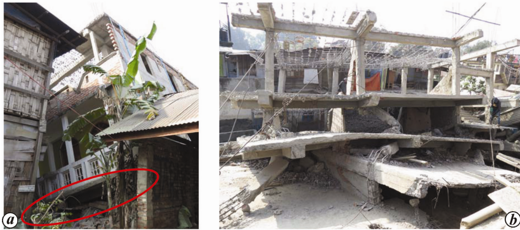
Figure 2. a , Collapse of a 3-storey building in Keishampat, Imphal; b , Collapse of a 4-storey building in Dewlahland, Imphal.
