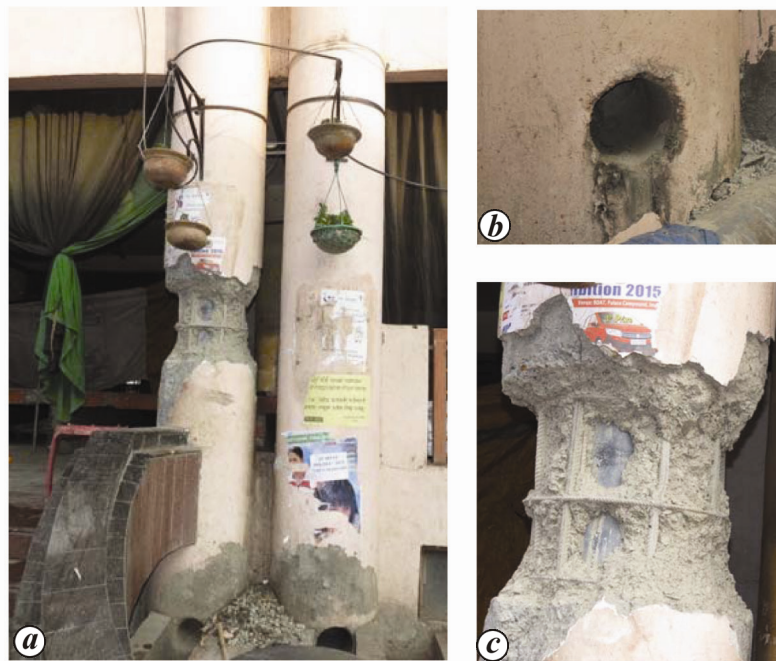
Figure 6 a-c. Concealed drain water pipes inside the exterior columns further compromised the confinement of core concrete in the circular columns of the buildings.
