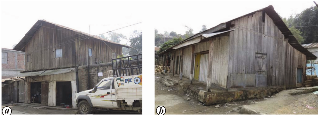
Figure 3. Good performance shown in traditional construction. a , 2-storey wooden house (known as Shing-Khim) at Dewlahland in Imphal; b , single storey Shing-Khim at Noney Bazaar near Epicentral region.
