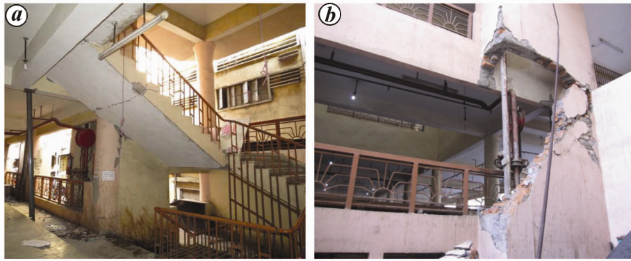
Figure 8. a , Severe damage to waist slab of RC staircase in Laxmi market; b , severe damage to masonry infill walls.
