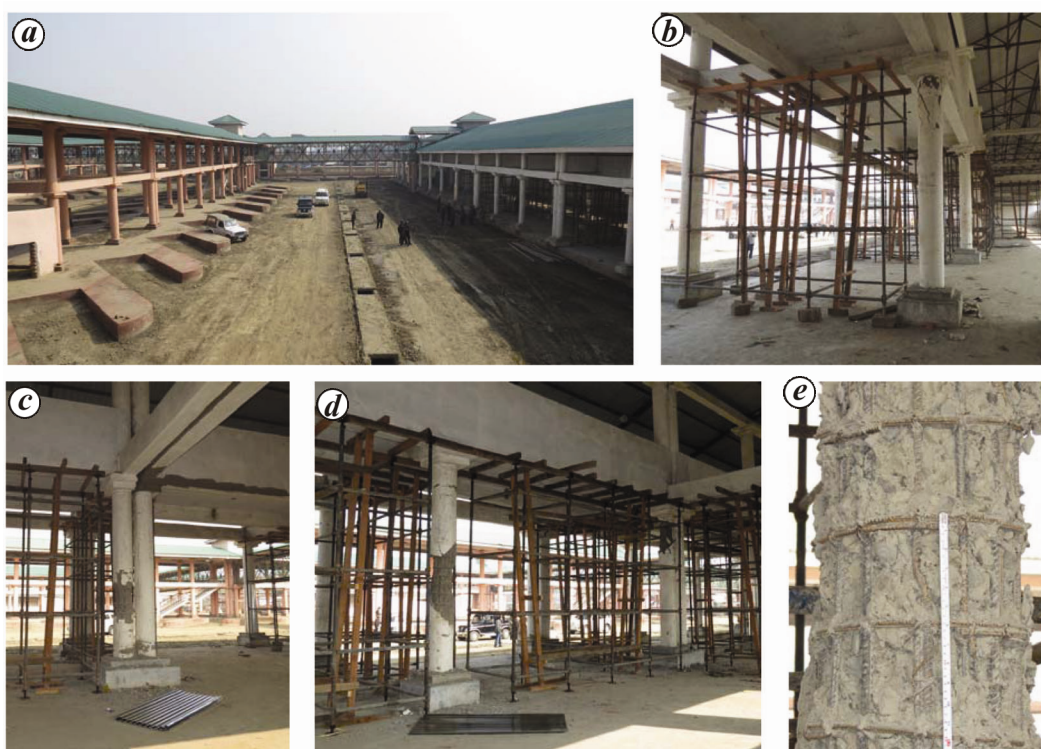
Figure 9. a , A view of Inter-State Bus Terminal at Imphal; b-d , severe damage to RC columns; e , non-ductile detailing in columns.
