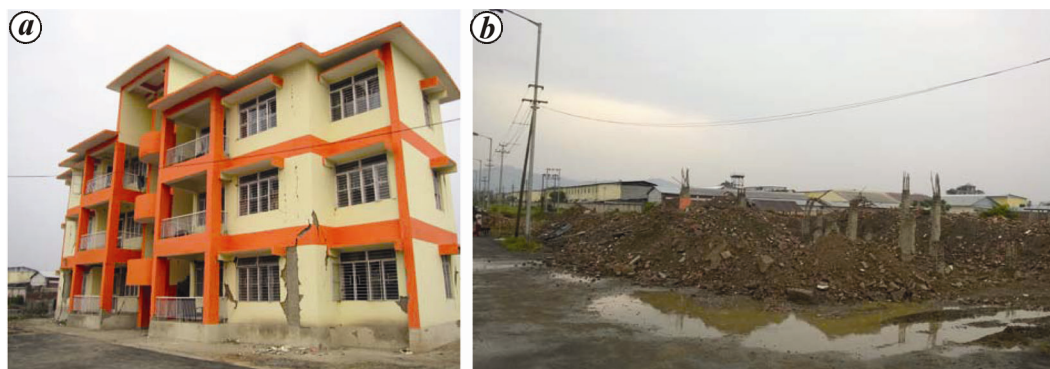
Figure 12. a , Minor to moderate damage experienced by staff/coach quarters in SAI complex; b , View of demolished quarters after three months.
