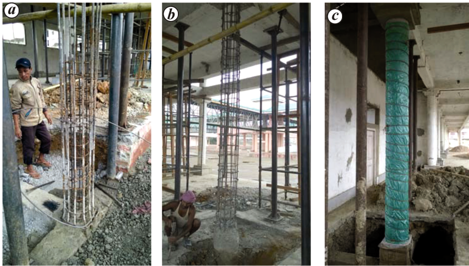
Figure 10 a, b . Retrofitting of RC column by replacing circular ties with helical reinforcement and addition of longitudinal bars along with ties in the existing concrete core; c , view of retrofitted column wrapped with plastic sheet for curing.
