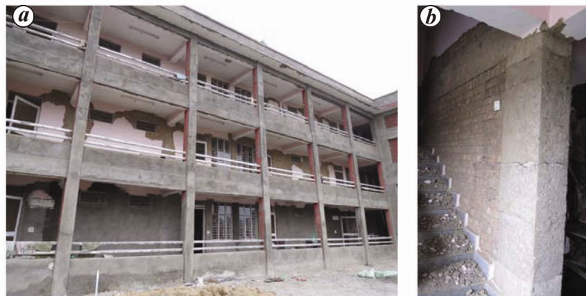
Figure 11. a , Damage experienced by hostel building in SAI complex; b , repairing of crack with plaster reinforced with steel wire mesh.
