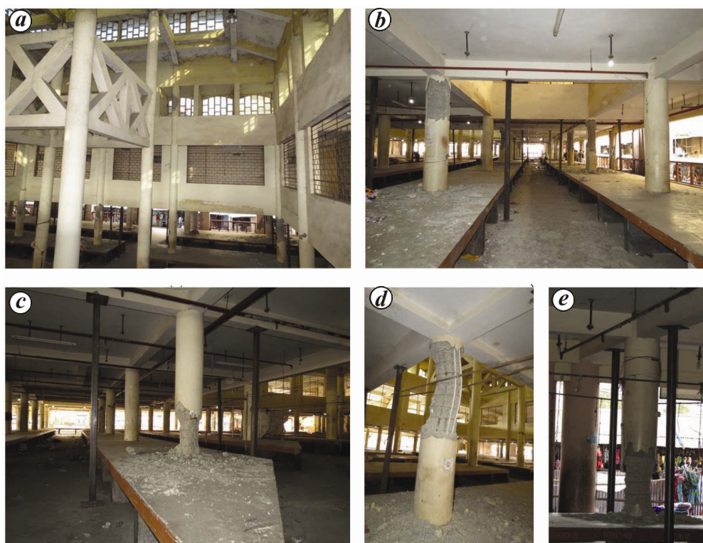
Figure 5. a , Soft first storey in Laxmi Market; b-e , severe damage to the RC columns of Laxmi and New Market.
