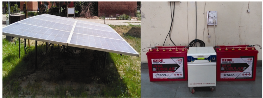
Figure 2. Solar photovoltaic system with power control unit for cold storage.
