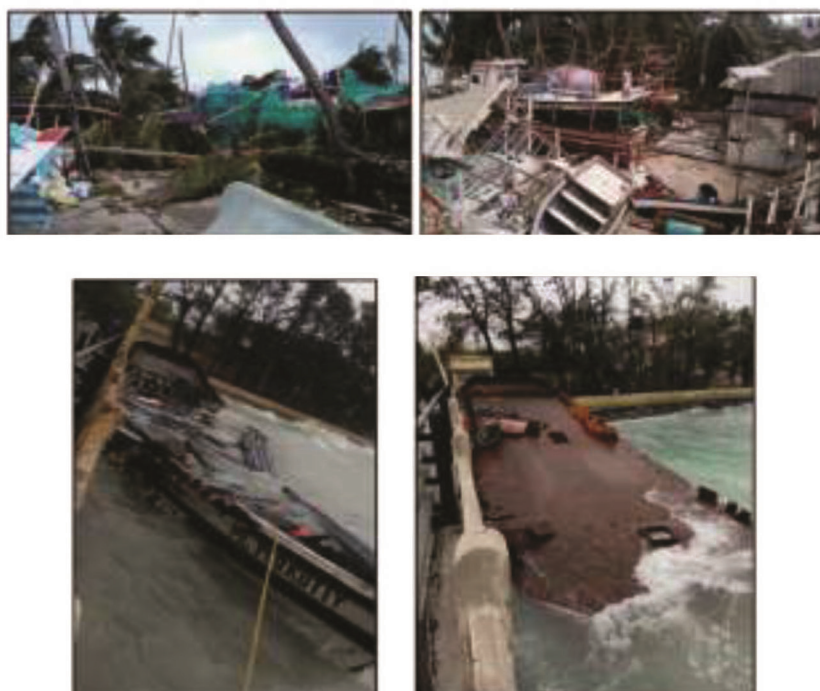
Figure 2. Photographs illustrating damaged boats and infrastructure in the Minicoy Island during the cyclone Ockhi .
