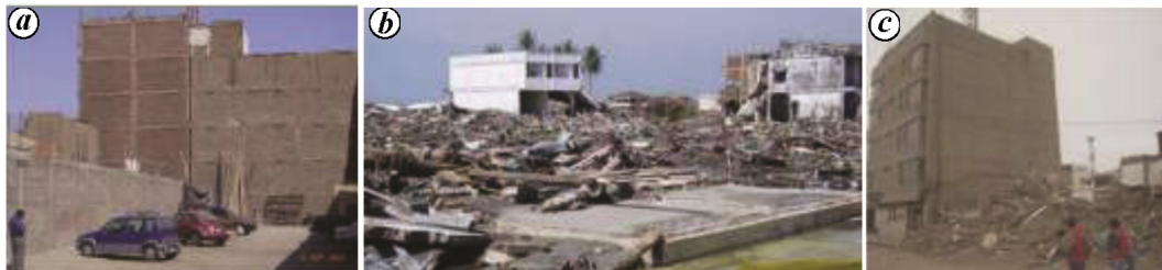
Figure 3. Good performance of CM construction in earthquakes. a , Six-storey confined masonry building in Ica, 2007 Peru earthquake 4 . b , No damage to confined masonry buildings, while collapse of other masonry buildings in El Salvador, 2001 San Salvador earthquake 5 ; c , Six-storey confined masonry building remained undamaged in 2007 Pisco (Peru) earthquake 6 .
