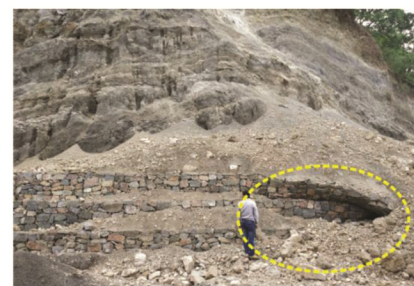
Figure 1. Deformed gabion wall along National Highway-58 near Rishikesh, Uttarakhand, India.
