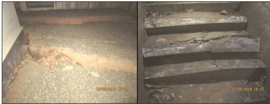
Figure 6. Damages in houses and surroundings due to landslide at Keerithodu in Kanjikkuzhy village.
