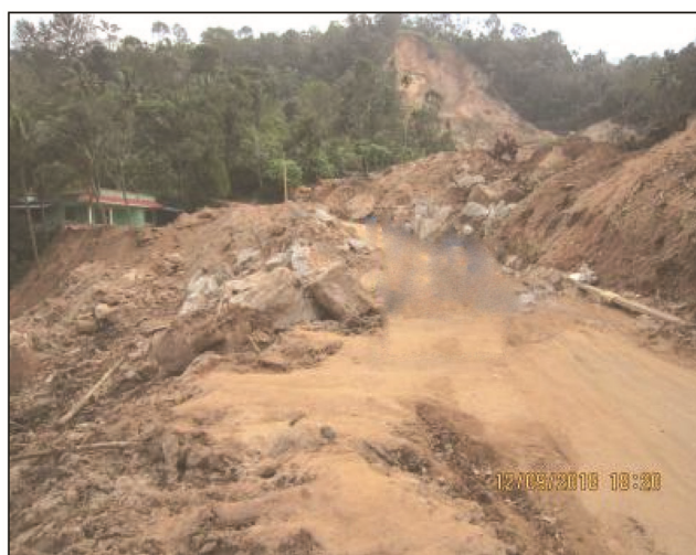
Figure 5. Landslide at Chittadikavala in Upputhodu Village.
