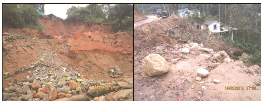
Figure 14. Landslide at Devikulam near Public Health Center (PHC) at Kannan Devan Hills (KDH).
