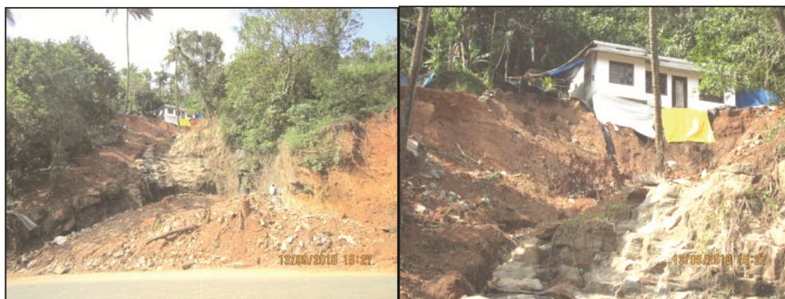
Figure 10. Landslide at Koompanpara, Mannamkandom village.
