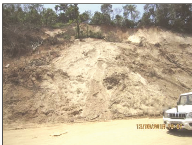
Figure 8. Landslide at Panniyarkutty in Konnathady village.
