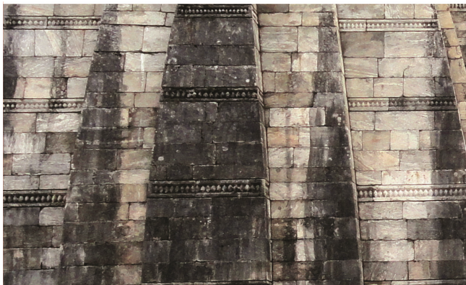
Figure 9. Blackish biofilm growing on the exterior surface of the temple after the flash floods encountered.
