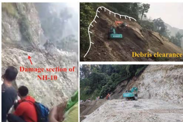
Figure 2. Road condition after the landslide. (Source: Fastest Fast Sikkim YouTube channel and East Mojo newspaper.)
