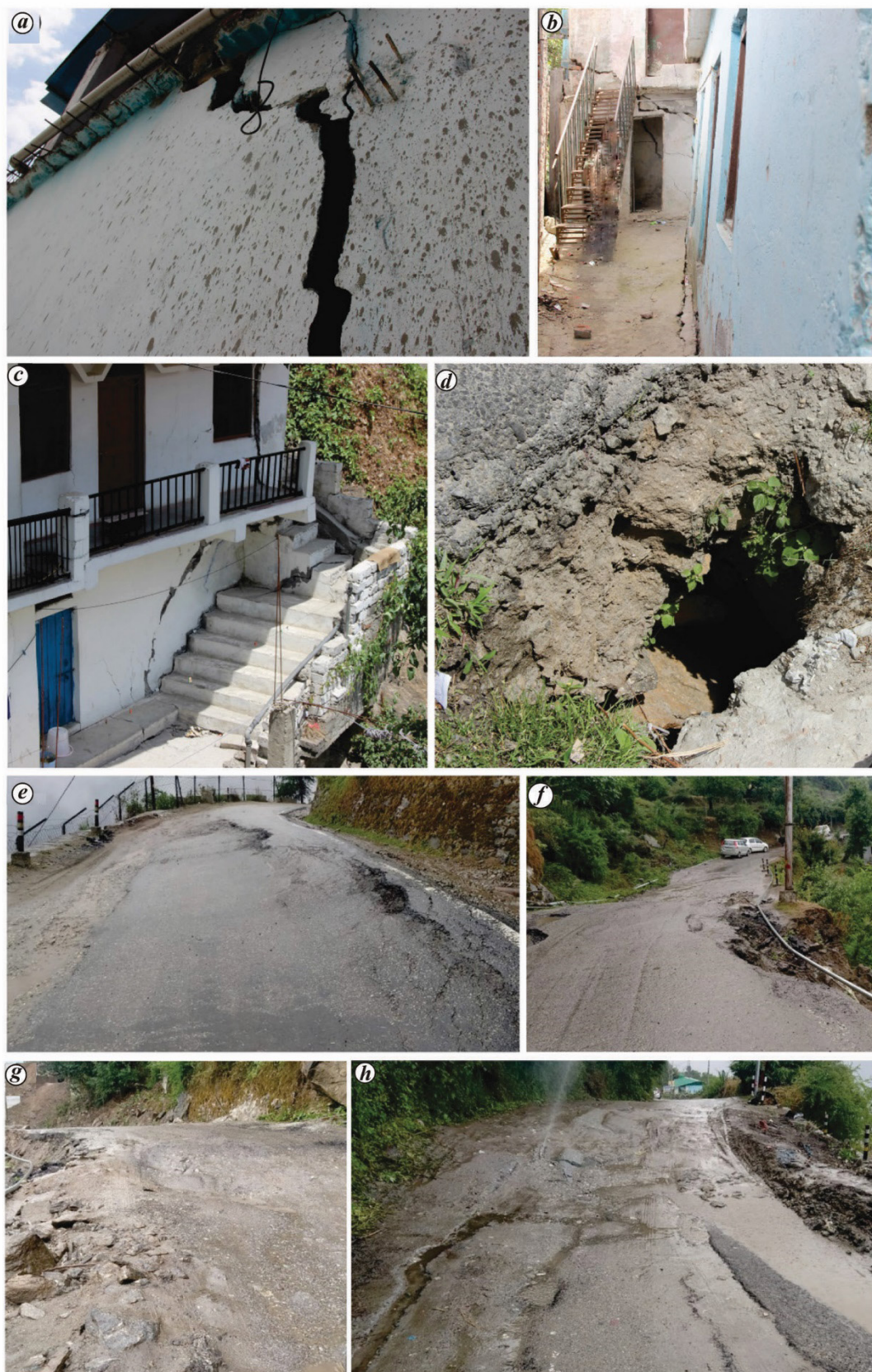
Figure 5. a–c , Damage caused to houses in the Chawani Bazar area (Badrinath road) due to continuous soil creeping. d , Potholes on the alluvium have become a regular feature, and are one of the reasons for eroding and transporting the fine matrix of the landslide deposits, thus creating caverns. e–h , Few segments of Joshimath–Auli road which are undergoing subsidence (photograph courtesy: Atul Sati).
