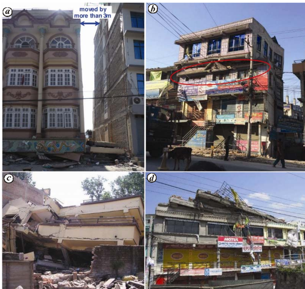
Figure 12. a , Open ground storey failure of four-storey building in Sitapaila, Kathmandu, ( 27^{\circ}42'42'' , 85^{\circ}16'58'' ) and ( b-d ), pancake collapse of single and multiple floors of commercial and residential buildings ( b , Machha Pokhari – 27^{\circ}44'06'' , 85^{\circ}18'20'' ; c , Sitapaila – 27^{\circ}42'36'' , 85^{\circ}16'59'' ; d , Kalanki Bus Stop – 27^{\circ}41'47'' , 85^{\circ}16'54'' ).
