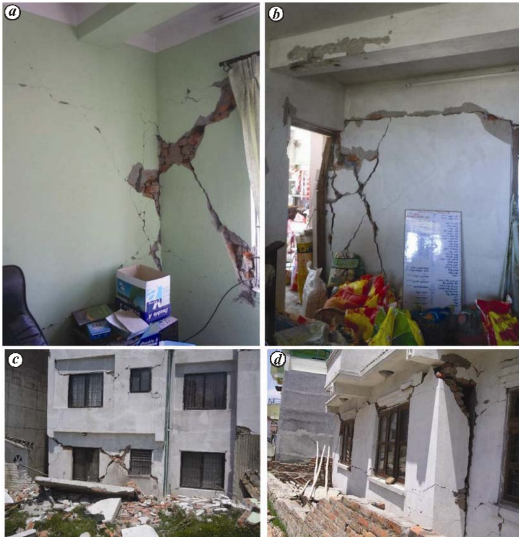
Figure 11. Various structural defects in newly constructed residential buildings in Kadhka Gaon ( 27^{\circ}41'43'' , 85^{\circ}15'53'' ): (a) Absence of column at the intersection of two walls. (b, c) Damage to the wall panel due to absence of confinement all around the openings. (d) Projection of masonry wall beyond the column grid line.
