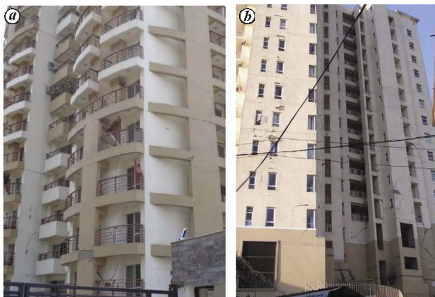
Figure 13. Typical damage to masonry infill in tall RC frame buildings: ( a ) 17-storey apartment building in Patan ( 27^{\circ}39'02'' , 85^{\circ}19'55'' ) and ( b ) 14-storey building in Kathmandu ( 27^{\circ}44'21'' , 85^{\circ}19'27'' ).
