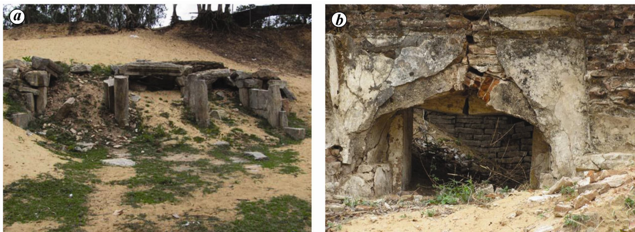
Figure 10. a , Dilapidated stone structure (possibly forming a part of an annexe temple) recovered from under the sand dune. b , Fractured and sagged gate-like structure made of brick. Both the structures are located within the compound of Kirtinarayan temple.
