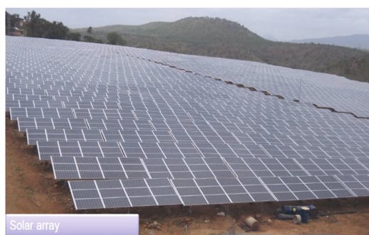
Figure 9. The 5 MWp solar PV power plant of Karnataka Power Corporation Limited.
