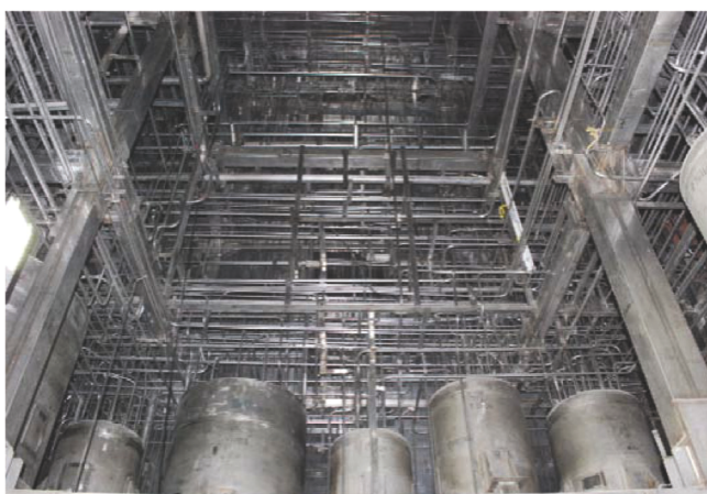
Figure 8. A view of complex stainless steel process piping inside shielded cells in Demonstration Fast Reactor Fuel Reprocessing Facility.
