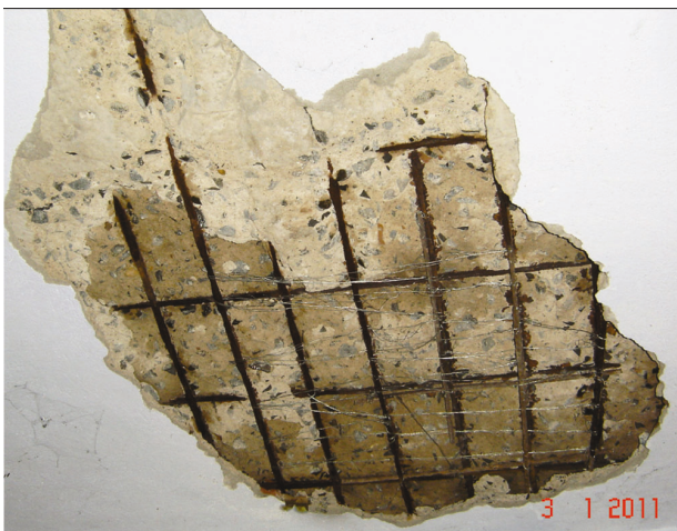
Figure 4. Damaged ceiling of a new building due to rainwater leakage.
