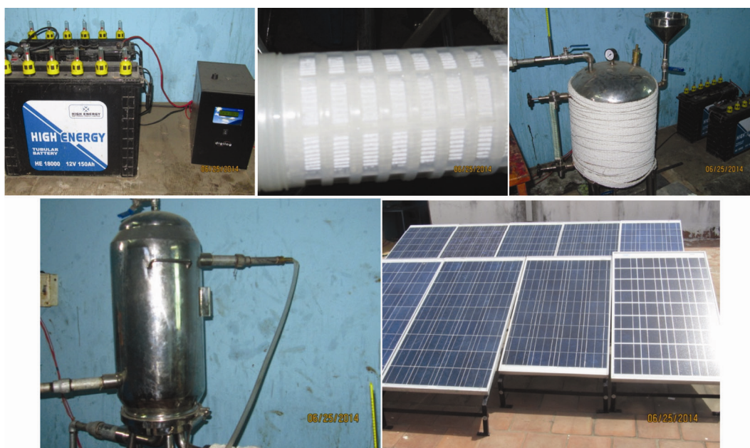
Figure 3. Photographs of solar PV powered membrane distillation components.
