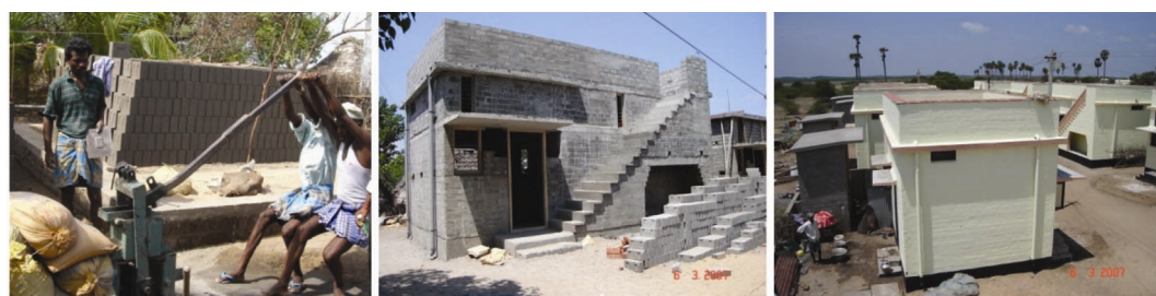
Figure 15. Compacted stabilized fly ash block production at construction site and the houses built.
