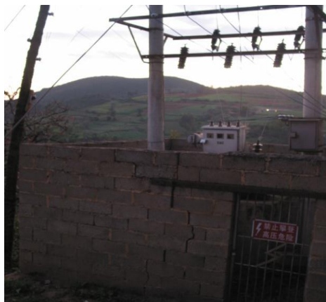
Figure 1 Cracks on the transformer resulting from landslide in Henggou Village
