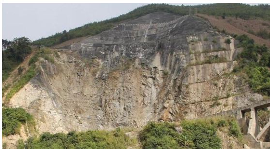
(a) Before reinforcement
