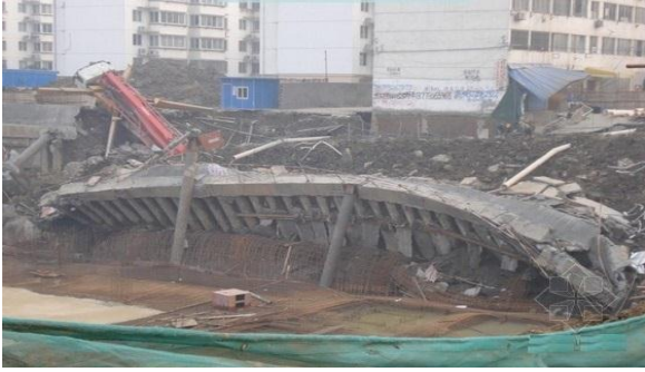
Figure 2: An example of unstable failure for a typical supporting structure of deep foundation pit
