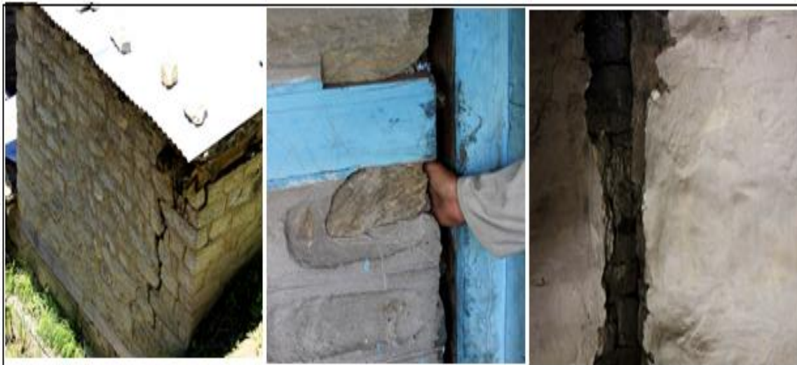
Picture 1. Cracks and Crevices due to the Blasting and Construction of HEPs in the Region
