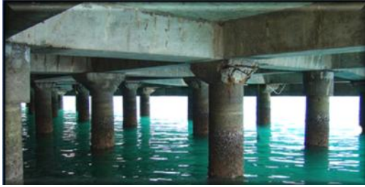
Figure 3: Marine structures under chemical deterioration
