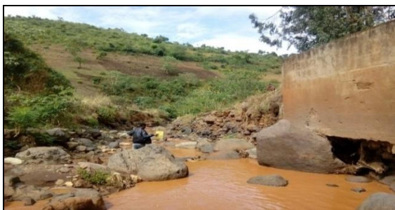
Fig. 5: Damages on downstream protection work at Awushoana SSI scheme
