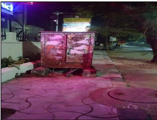
Figure 9: Electric Board obstructing the Footpath in Reach 2A
