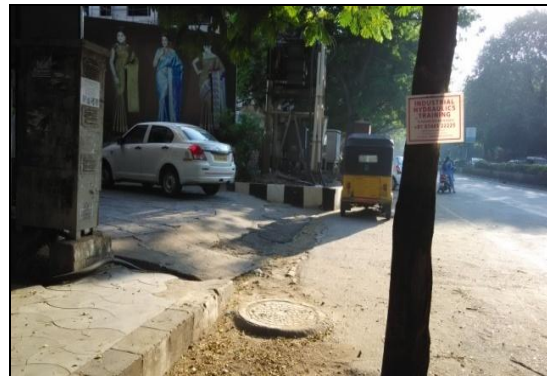
Figure 5: Raised Manhole Cover in Reach 1 B
