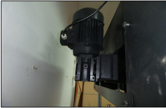
Fig.6: Three – phase motor
