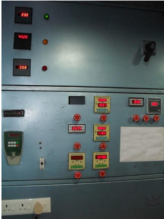
Fig. 9: Control Panel with different displays
