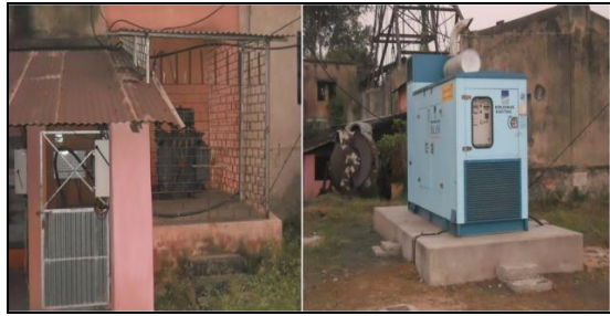
Fig. 4: 100 kVA transformer station and 125 kVA diesel generator
