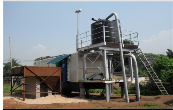
Fig. 7: Photograph of the caravan, inlet water pipelines and the overhead tank
