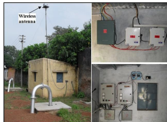
Fig. 3: Pump room with pump outlets, main switches and starters
