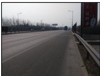
(a) Drawing of onsite road surface deformation
