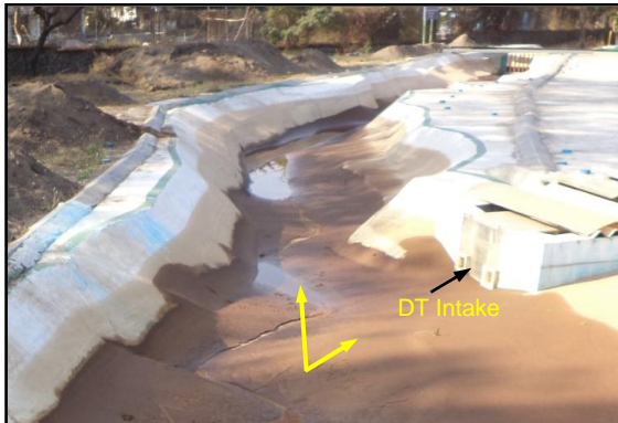
Figure 6: Deposition when DT is closed
