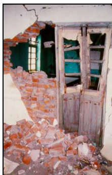
Figure 6: Out of plane failure in 1997 Jabalpur Earthquake (EERI, World Encyclopedia report, India, 6-5-2002)
