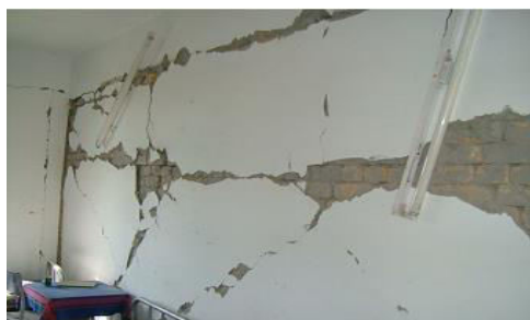
Figure 5: Flexural & shear cracks alongwith separation of wall from wall connection (S. H. Farooq, 2006)
