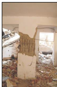
Figure 7: Shear failure in RC column (Jag Mohan Humar et. al., 2001).
