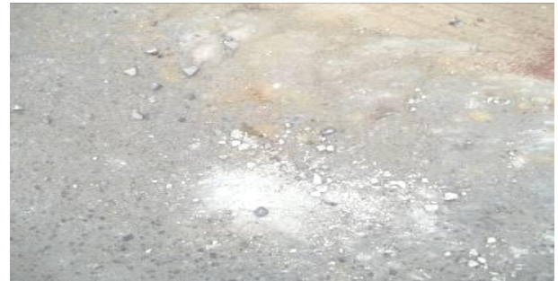
Fig. 2(b): Spalled asphalt road surface
