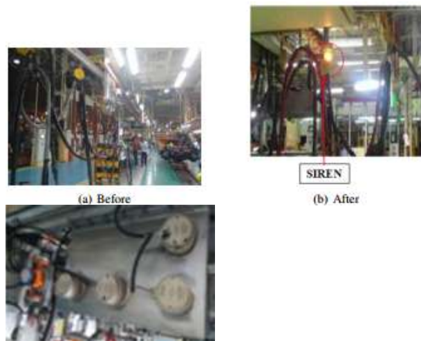
Fig. 4: Visual indicators and float switch usage (bottom)
