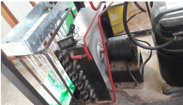
Fig. 3: Water sprayer ahead of condenser
