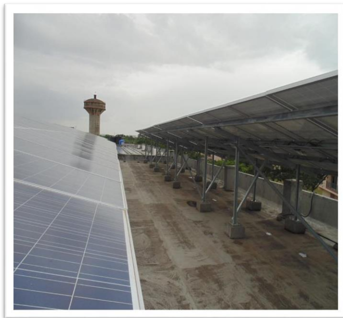
Fig 4(b): Side view of installed solar panels.
