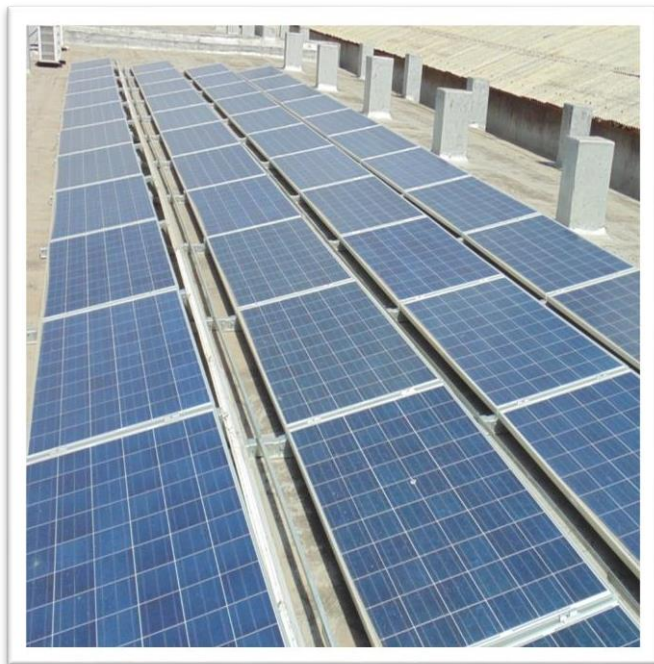
Fig 4(a): Top view of installed solar panel.
