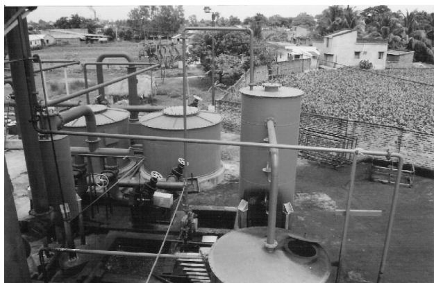
Fig 3: A typical 250 kwe gasifier unit of a rice mill
