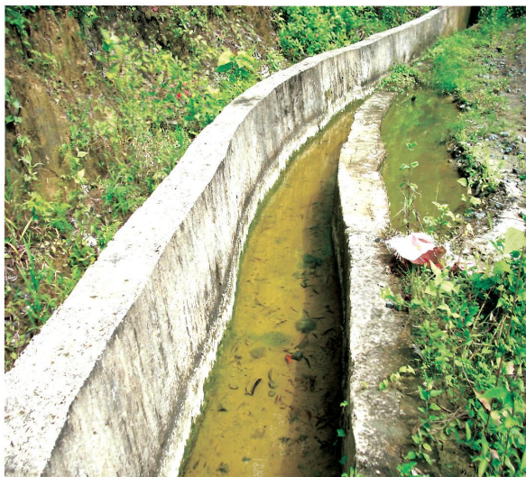
Rain water drainage on Laxmi Nagar
