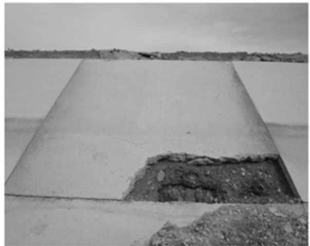
Figure 4. Failures in the concrete lining.
