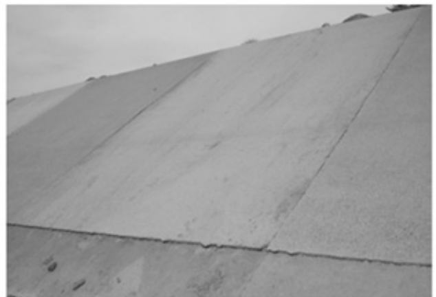
Figure 2. Crack, and uplift of concrete lining.
