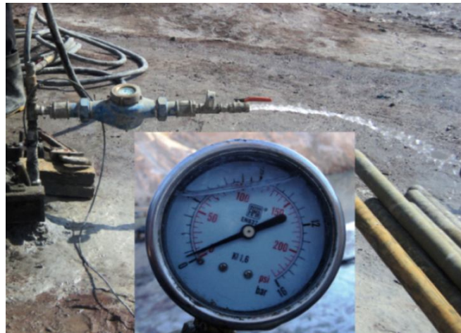
Fig. 4. Inner damage zone: This zone had the highest Water leakage ( Q=1\text{lit/s} , p=0.8\text{ bar} ).
