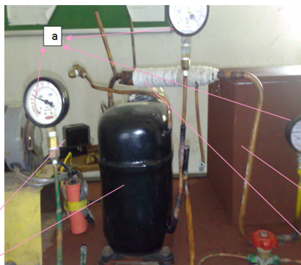
Plate 1. Reciprocating Compressor with Heat Exchanger set up
