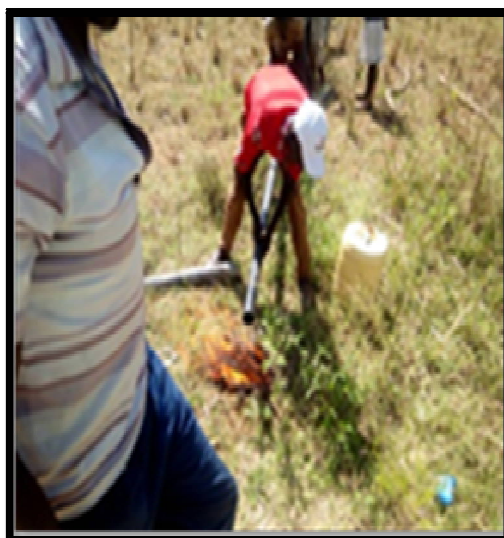
Figure 3: Hand Pump under Repair
