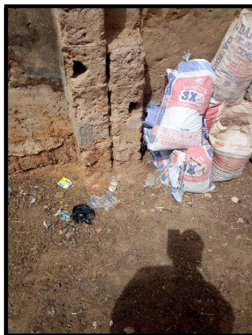
Figure 6: Showing the Real Feature of Deterioration of Structure in the Study Area
