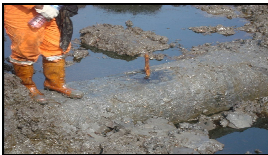
Figure 2: L A Segment of Badly Corroded, TNP in Bodo, Gokana LGA (Source: Zabbey, N)
